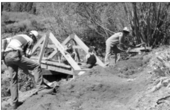
Volunteers installing one of the two new bridges in Negro Canyon along the Donner Rim Trail. To sign up for the 2006 season, call or email the Land Trust.
