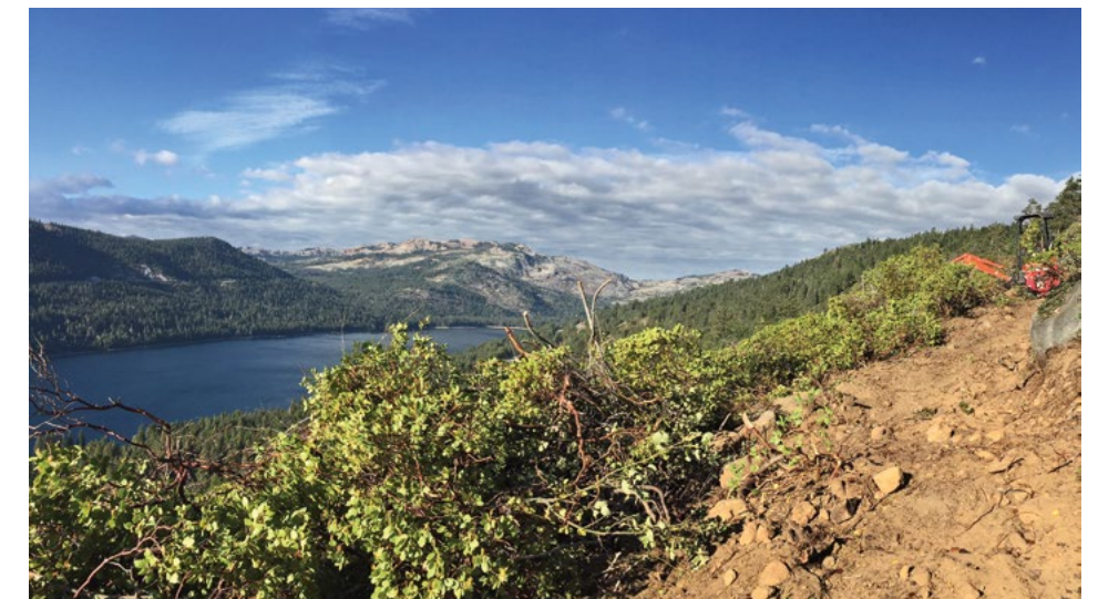
The view from the new section of trail under construction last summer.
