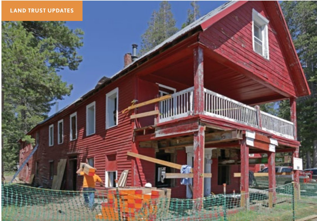
Last summer engineers shored up the Webber Lake Hotel and carefully lifted it off the ground to pour a foundation.
